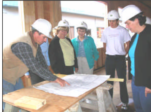
Bruce Young, Site Manager from Maddocks Construction describes plans to NONA staff during a recent tour of new building.
