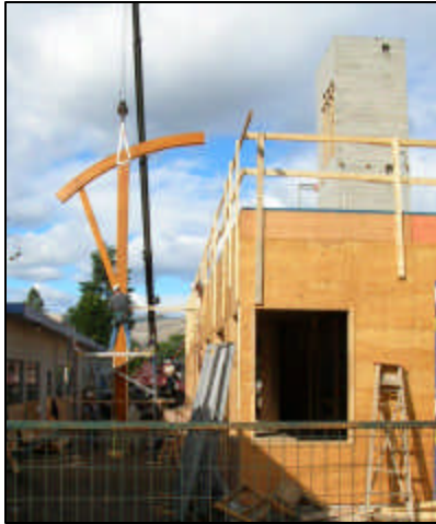
Bruce Young, Site Manager from Maddocks Construction, secures the first beam of our Centre's Entrance.
